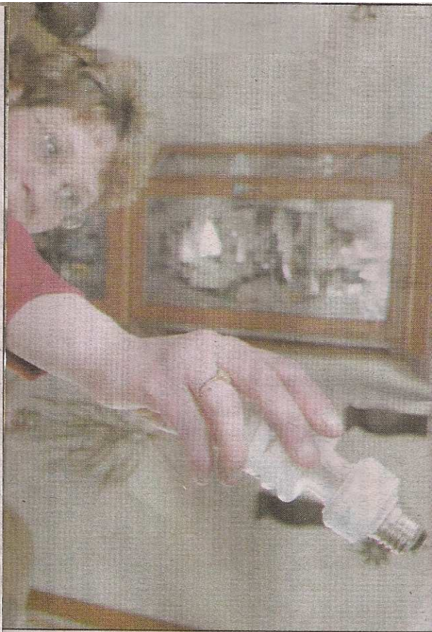
Marquette Township resident Dianna Truscott installs a compact fluorescent light bulb in a ceiling fan in her home Thursday. Truscott is one Habitat for Humanity homeowner to recently receive a box of CFLs. (Journal photo by Andy Nelson-Zaleski)
