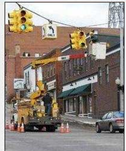
Marquette Board of Light and Power lineman Sean Seibert stands in a bucket lift as he replaces old traffic light bulbs with new LED lights at the corner of Washington and Third streets in Marquette in January 2008. The new lights have an extended life of 10 years and are more energy efficient. (Journal file photo)
